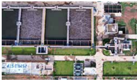
25 MLD STP, Jagdalpur, Chattisgarh
