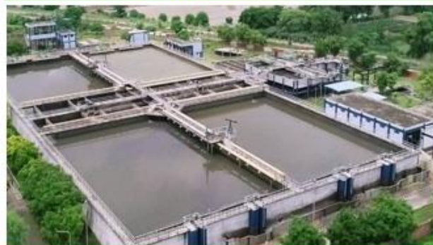
52 MLD STP at Bhatinda Punjab
