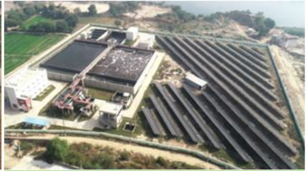
30 MLD STP Kota Rajasthan (includes solar plant)
